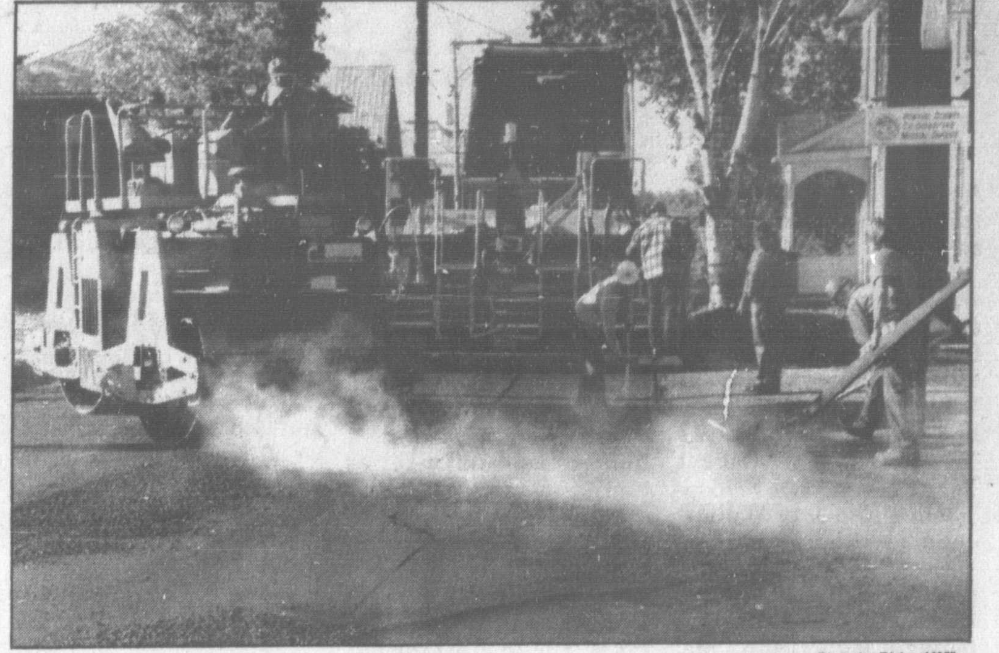
With steam raising from hot pavement on a cool autumn morning, workers applied new pavement to Highway 303 through Centre Street in Shawville on Monday, October 3rd.
