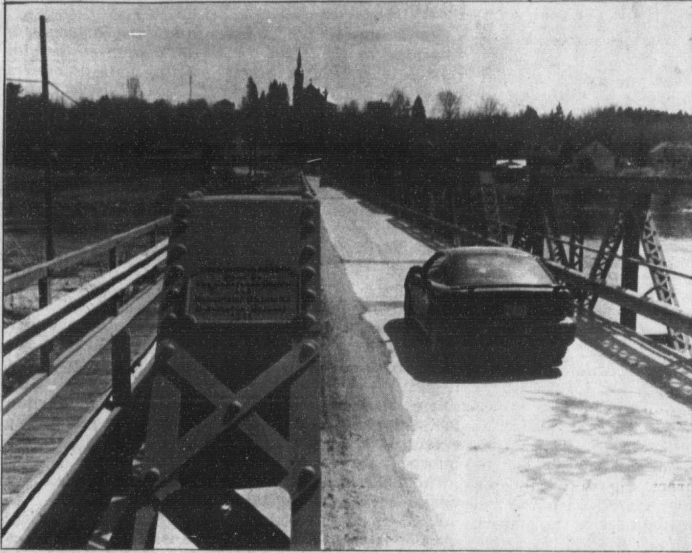
On May 17 the one-lane bridge in Chapeau, built in 1911, will be closed.
